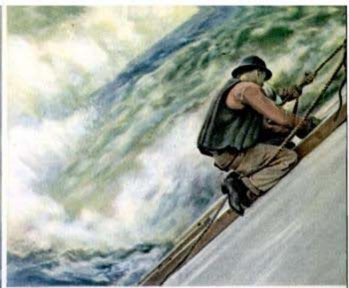
21248 Workman on safety line removes temporary construction material on lower face of the dam
